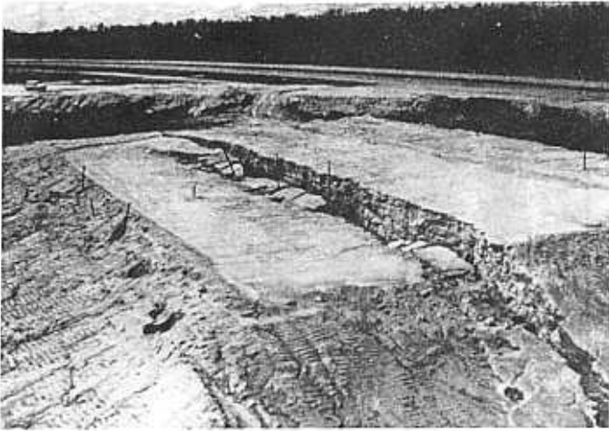
FIG. 2. View of Tensile Fracture of Compacted Fill
